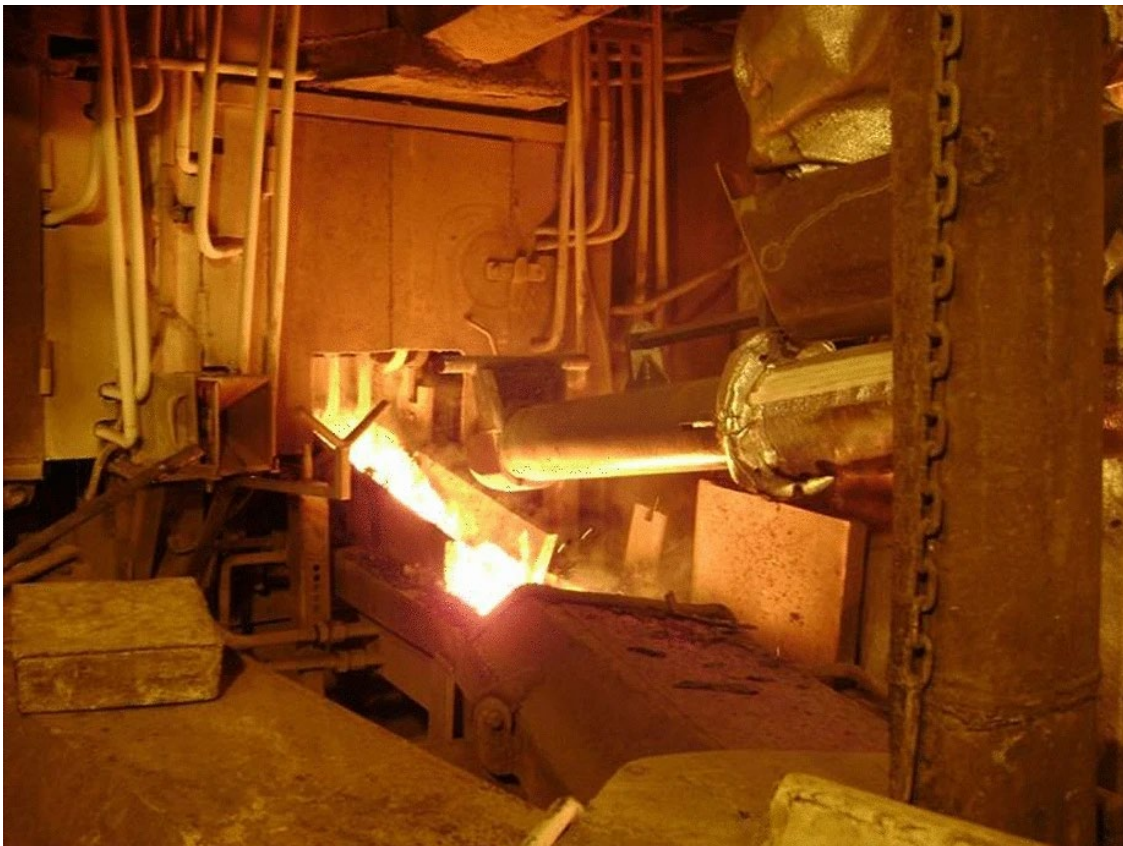
Figure 8: The MIRS automated, heavy-duty, ceiling-mounted furnace-tapping robot with exchangeable drill tools and plugging tools (e.g., mud gun), equipped with a heat-resistance suit. Source: [8]
